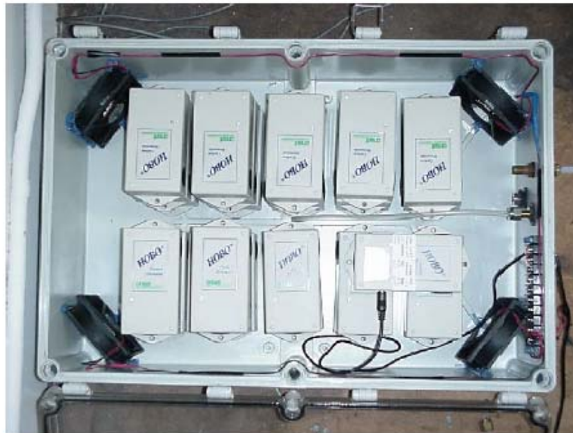
Figure 4-1. Chamber for Calibrating the Onset CO Analyzers
